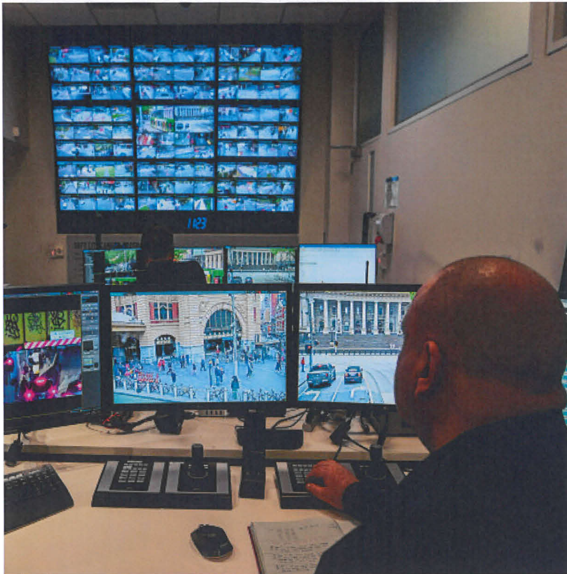
Looking for trouble. Inside the monitoring room. CREDIT:JOE ARMAO
