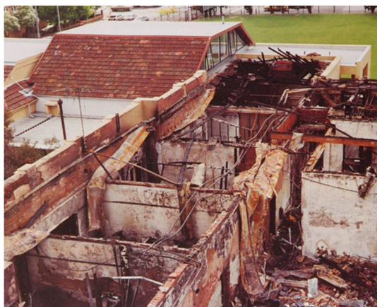
Figure 21. Photograph showing the West Wing destroyed by fire, 1989. (Source: Wesley College 2021)
