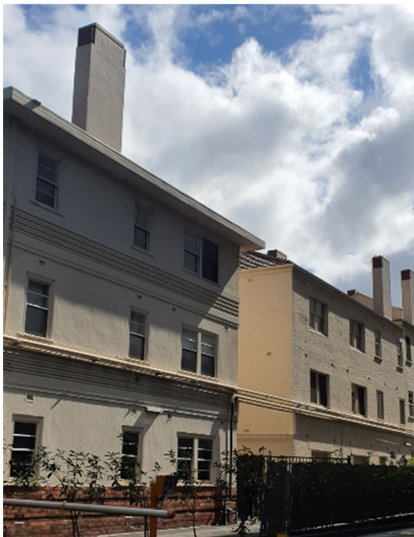
Figure 20. Southern side of the building showing the back of the building painted cream without render. (Source: GML Heritage 2021)
