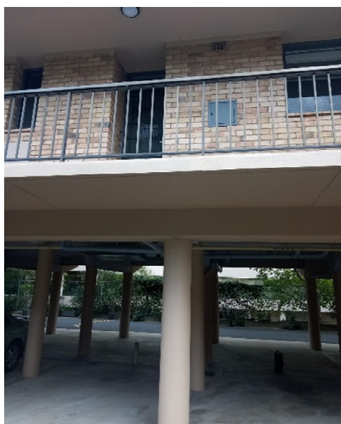
Figure 12. Metal balustrade to galleries above pillar to first floor base. (Source: GML Heritage 2021)
