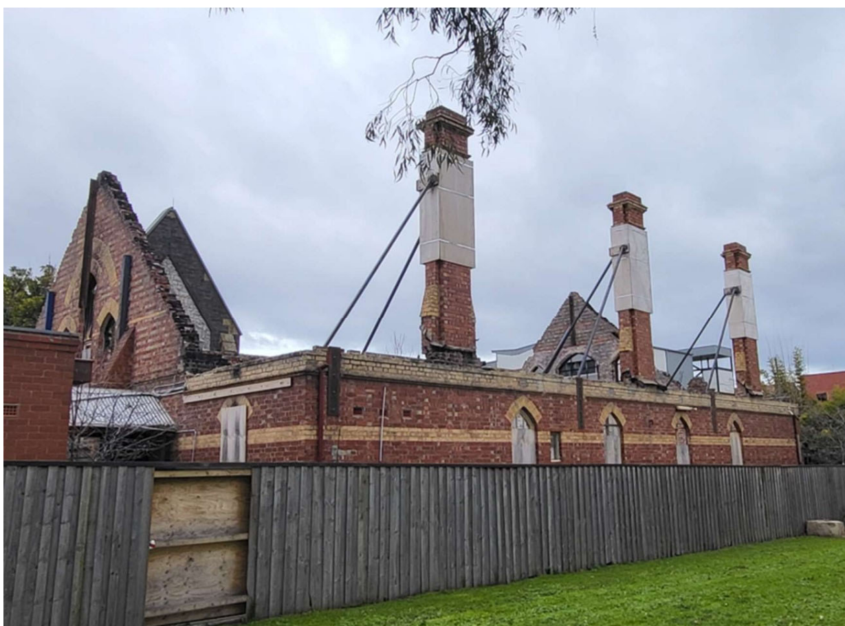
Figure 10. View of the 1884 Sunday school building from Fawkner Park after the fire event in May 2022 (Figure 7: Number 4). Note the original elements including the chimneys and pointed arched openings remain . (Source: N Schmeder 2023 City of Melbourne 2023 GML Heritage 2021 )
