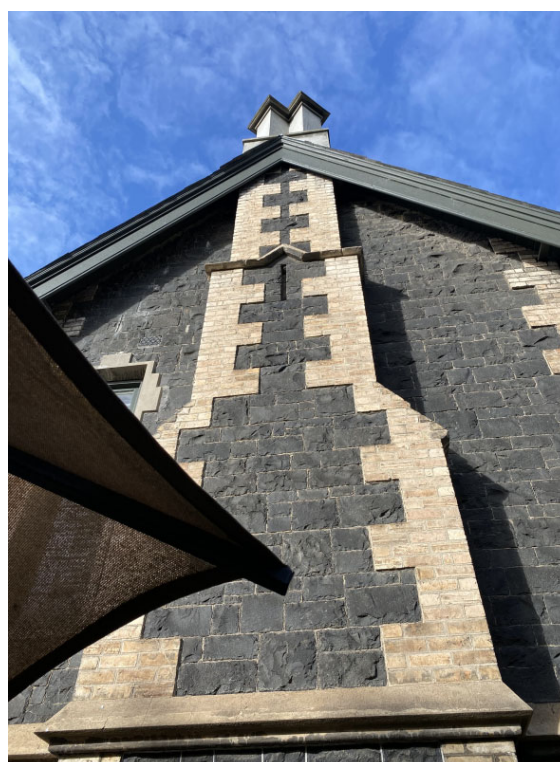
Figure 8.- The chimney stack with quoining on the northern elevation of the vicarage. (Source: GML Heritage 2021)
